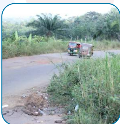
Images of poorly constructed Isieke - Ajatah Road in Umuahia North LGA, Abia State.
