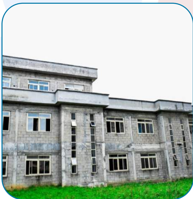
Images of uncompleted Niger Delta Regional Hospital (Cardiovascular) in Port Harcourt, Rivers State.
